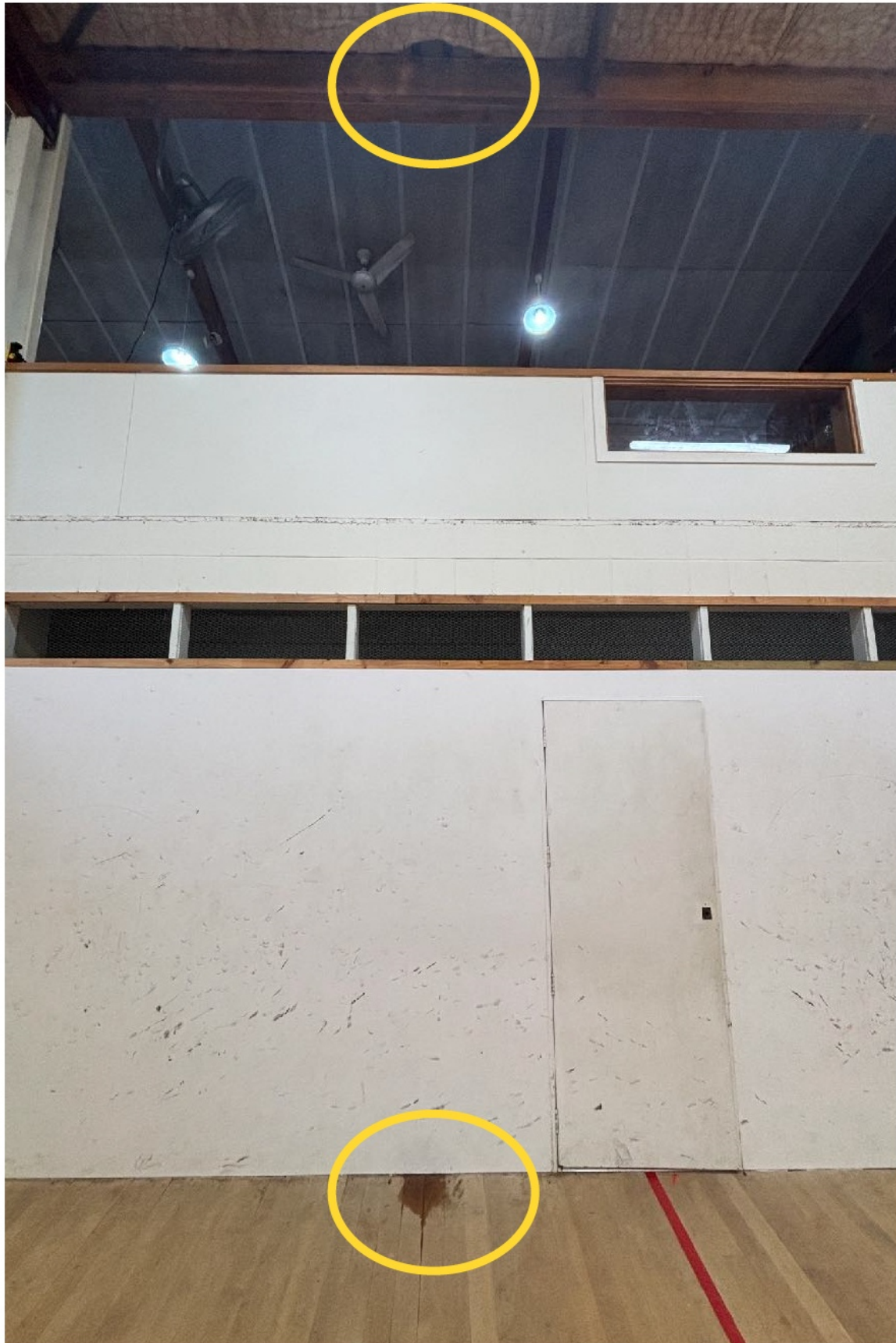
Example of a recent mild leak. The top circle is the bottom of the damaged wall shown in the previous pictures. Rain then drips down onto the back of the courts.
