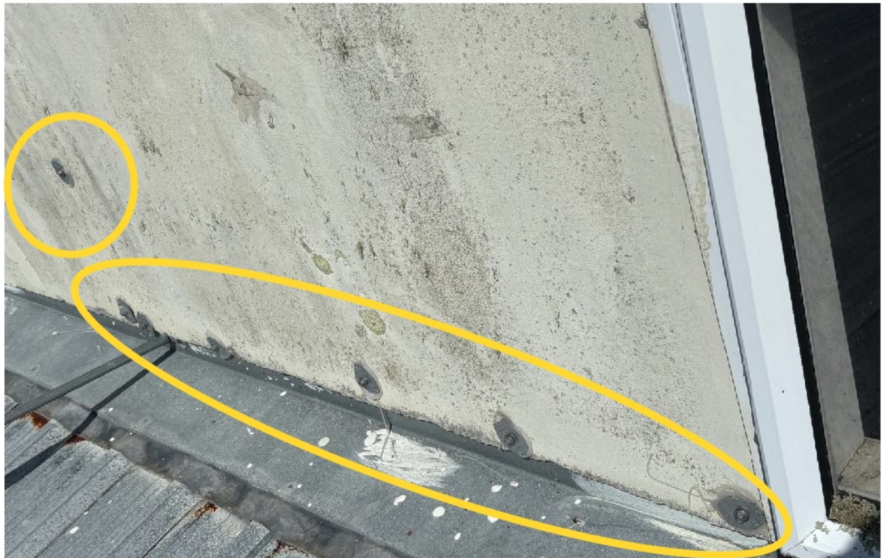
Examples of remedial patches applied to damaged areas of Hardie Board to slow in ingress
