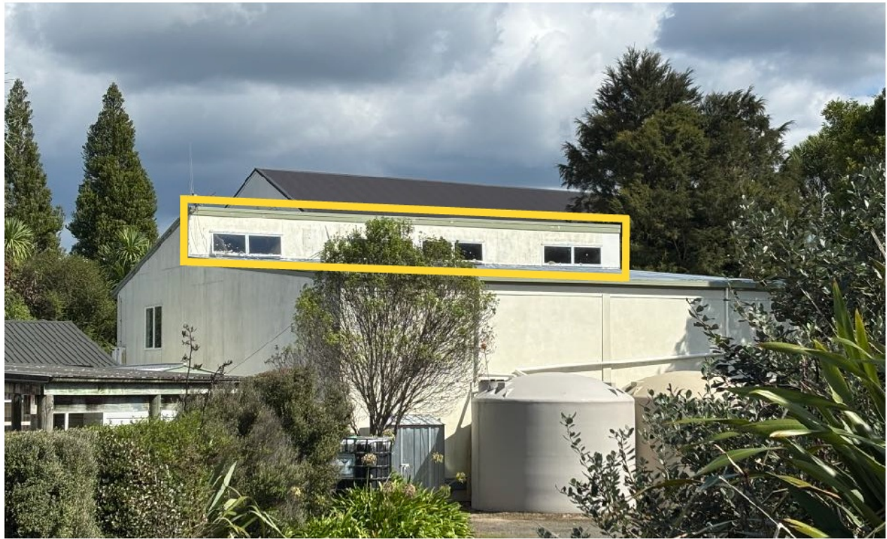
The framed area is the section of wall requiring re-cladding
