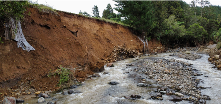
The landslide damage at Te Tahi reservoir.
