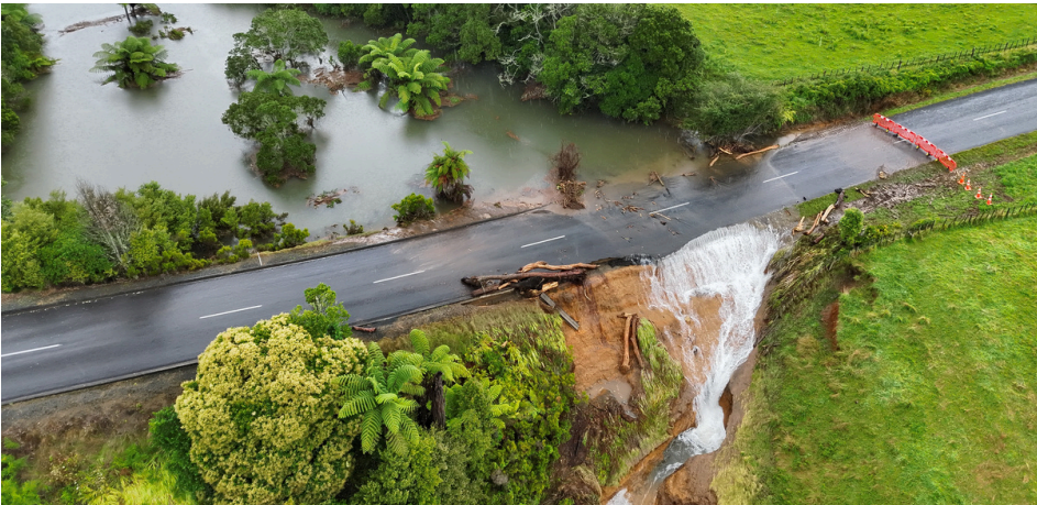
Corcoran Road in Te Pahu is closed with risk of collapse, with residents downstream evacuated.
