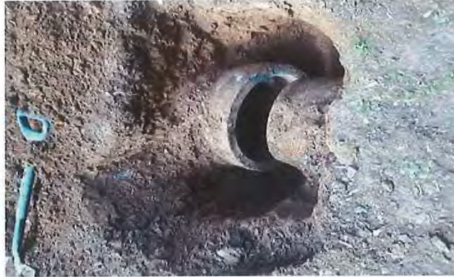
Figure 1. An example of disconnected sections of culvert piping.
