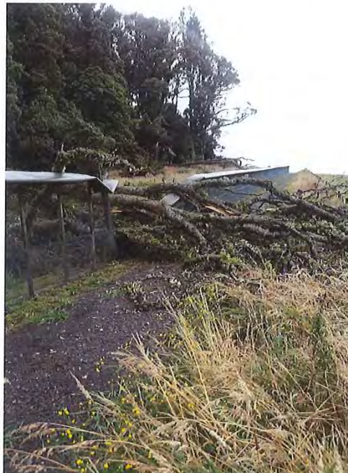
Figure 5. Tree fall causing major damage to the pest-proof fence.
