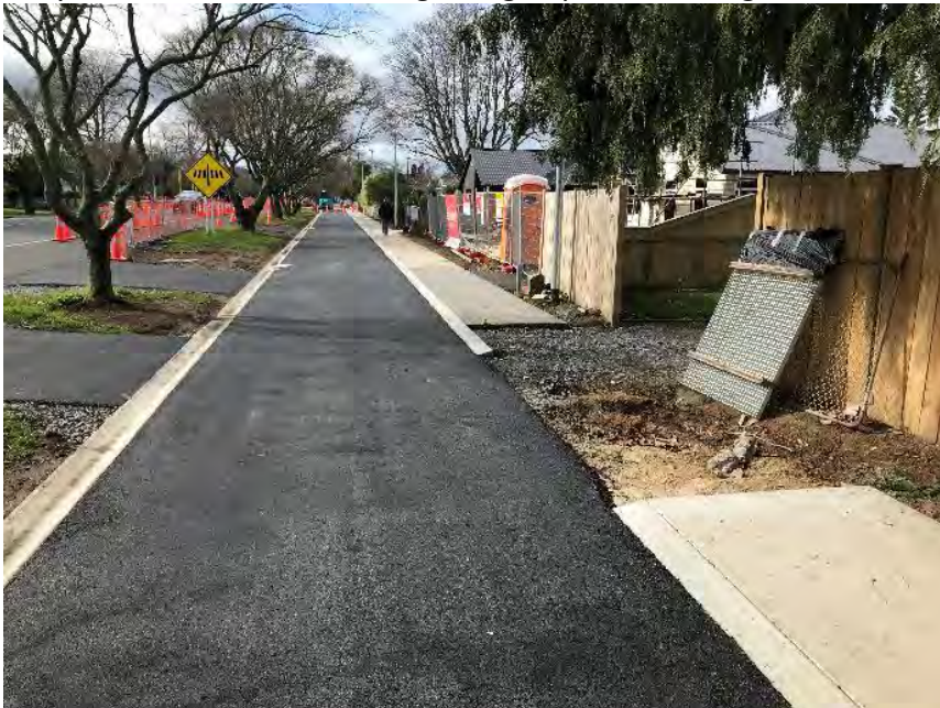
Cycle path ready for road marking. Special fibreglass panel standing against the fence is to be laid over shallow tree roots to complete the pedestrian footpath.
