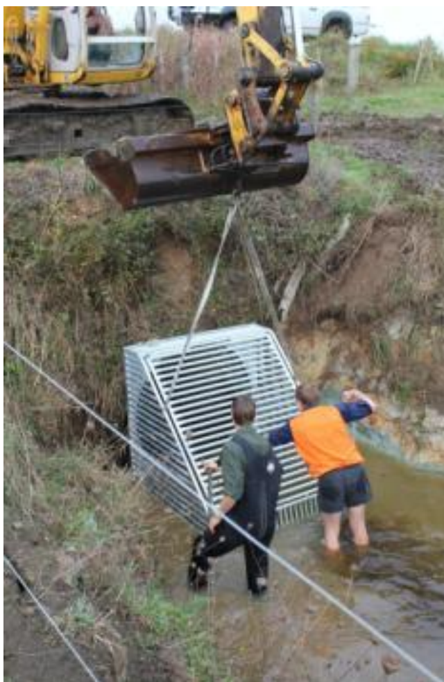
Koi carp barrier being lifted into place at Lake Ohinewai. This will enable adult koi to leave the lake, but not return. (Photo credit: J Gumbley, DOC)
