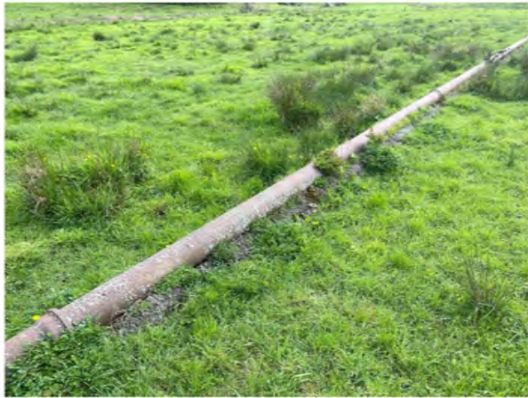
Pipeline situated on concrete foundation (Type 1)
