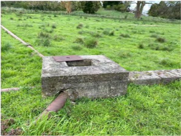
Concrete chamber connecting all four pipelines (Type 7)
