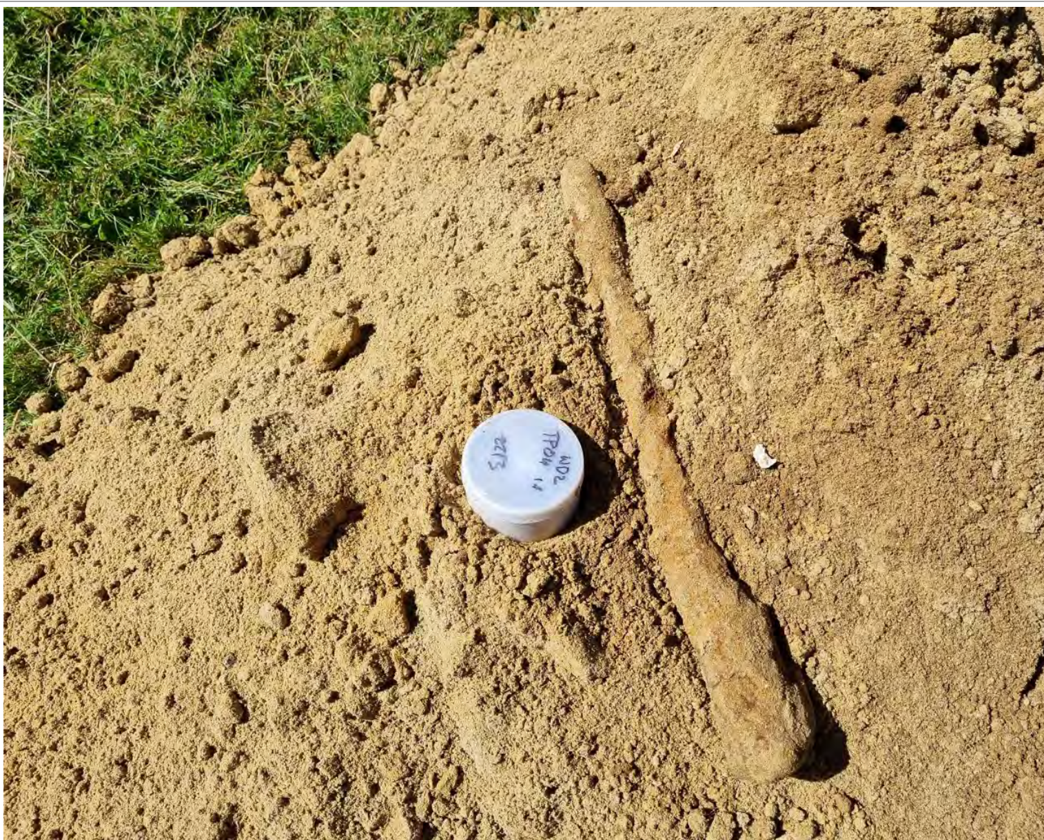
Photo 2 – WD2_TP 04: Metal pipe
