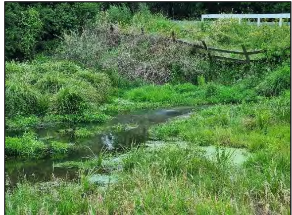
Photo 6: Pooling above Culvert 1.
