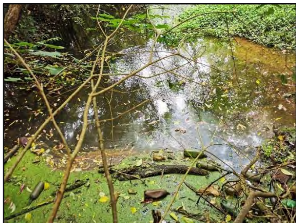
Photo 7: Downstream Culvert 2. Pooled water and debris visible.
