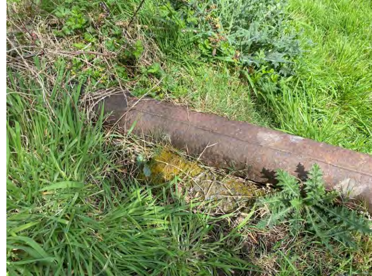
Pipeline situated on concrete foundation
