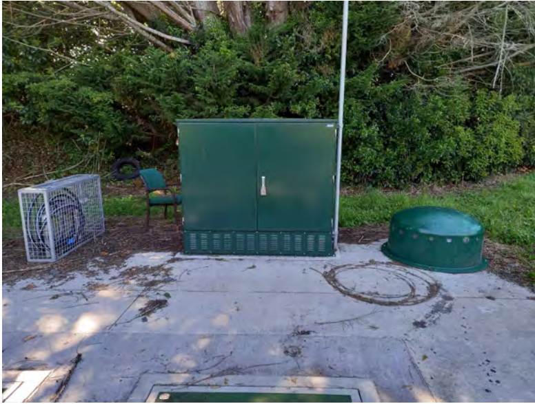
Wastewater Pump Station (WWPS)
