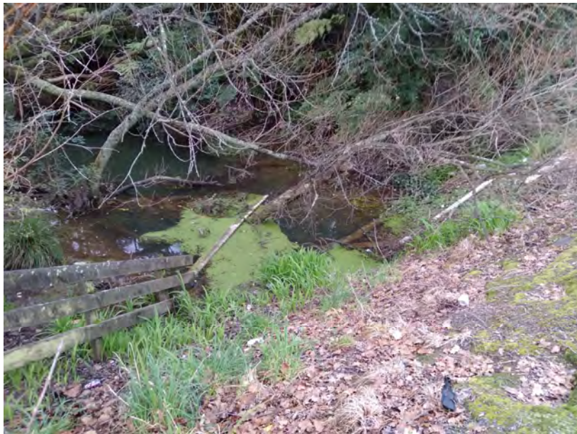
Culvert 1 Outlet – note extensive debris/windfall
