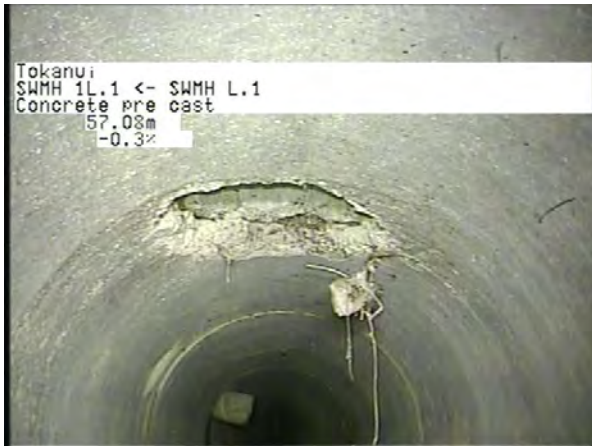
MH L.1 To MH 1L.1_86a0788c-11dd-40f7-a6c0-3777bbc11132_20230404_1 21725_361.jpg, 00:15:28, 57.08m
