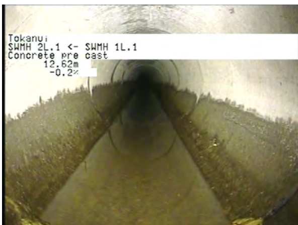
MH 1L.1 To MH 2L.1_093e2240-aeb3-44ec-962a-a4ac91c675dd_20230404_1 25730_151.jpg, 00:04:10, 12.62m
