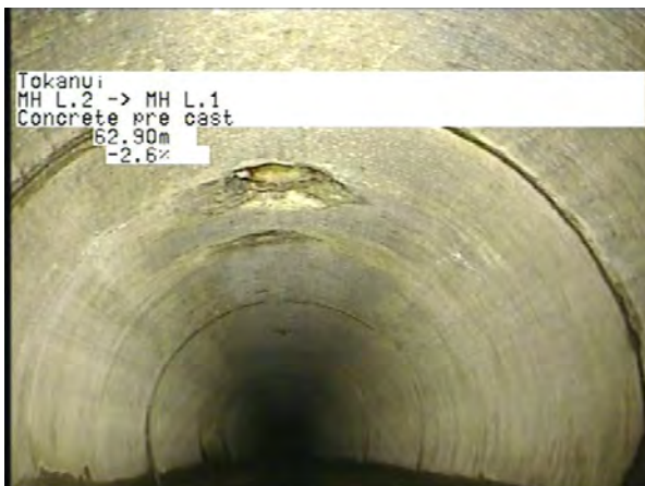
MH L.2 To MH L.1_849fab06-2ce5-4837-b552-7d49813f3271_20230328_120204_715.jpg, 00:20:10, 62.90m
