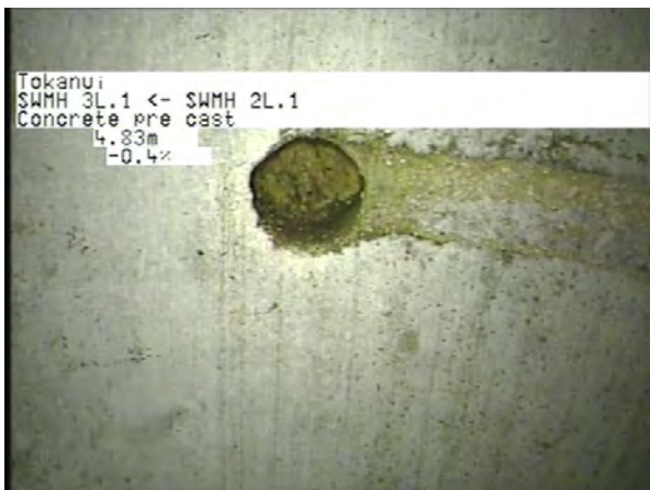
MH 2L.1 To MH 3L.1_9af431fd-b2b1-4d42-a45b-882d6635cdf3_20230406_11 5851_257.jpg, 00:01:57, 4.83m
