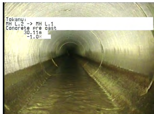
MH L.2 To MH L.1_ecea2b43-d4e0-4411-be2f-42ea484c9973_20230328_114733_026.jpg, 00:08:38, 30.11m
