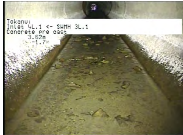
MH 3L.1 To Outlet 4L.1_8e005ace-6982-4f74-a075-611227db762a_20230406_1 24600_011.jpg, 00:01:16, 3.62m
