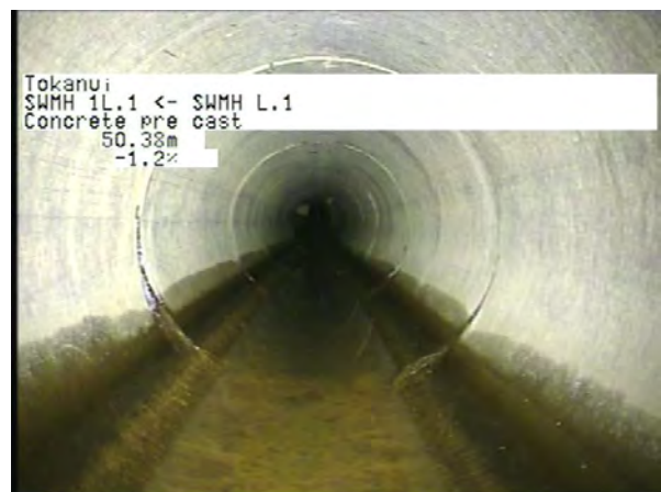
MH L.1 To MH 1L.1_67567631-e148-4c01-88fd-9c6bdd18b35a_20230404_1 21553_955.jpg, 00:14:08, 50.38m
