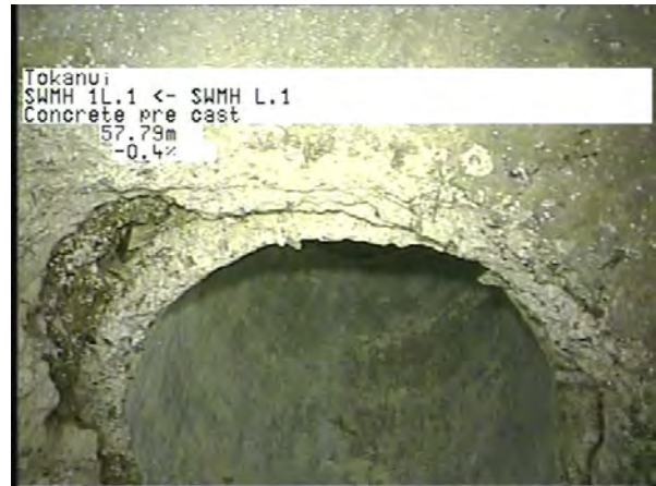
MH L.1 To MH 1L.1_42f8a8e7-9c5f-4050-acd7-894a60ad9256_20230404_12 1758_258.jpg, 00:15:44, 57.79m
