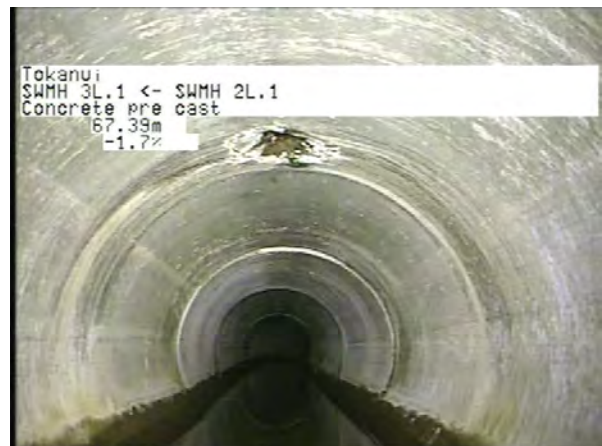
MH 2L.1 To MH 3L.1_f8a626dc-c15d-4079-b907-47acf5c79cff_20230406_122 127_184.jpg, 00:21:48, 67.94m
