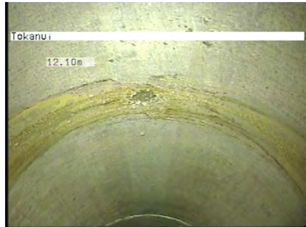
MH L.3 To MH L.4_03d758d2-c9f0-4aed-bd14-6ea585a74467_20230404_09 3442_339.jpg, 00:05:27, 12.10m
