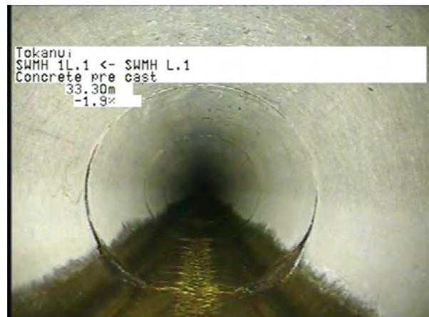
MH L.1 To MH 1L.1_04a8f97b-4bad-48b7-8a96-fea918bddee7_20230404_12 1146_371.jpg, 00:10:19, 33.30m
