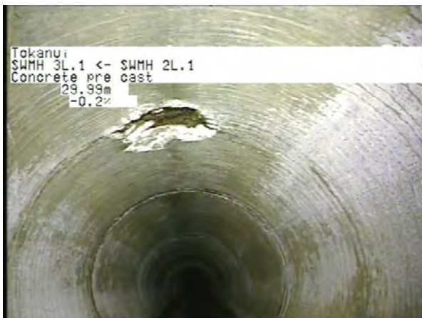
MH 2L.1 To MH 3L.1_eba0790a-3924-4b26-907a-3cd8429df09d_20230406_1 20730_087.jpg, 00:09:52, 29.99m
