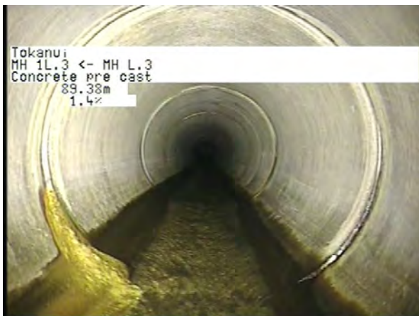
MH L.3 To MH 1L.3_6fc0d206-46fe-4ded-84f3-3717a3a2e390_20230404_10 5632_934.jpg, 00:24:01, 89.38m
