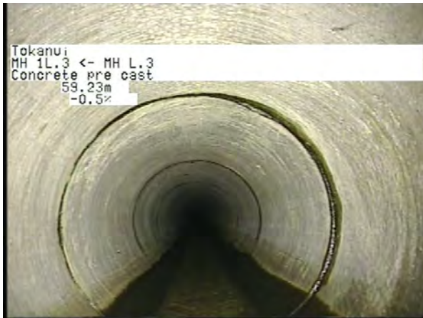
MH L.3 To MH 1L.3_dbe0252b-adad-401c-83c7-f555bd97aa7f_20230404_10 4742_860.jpg, 00:16:48, 59.23m
