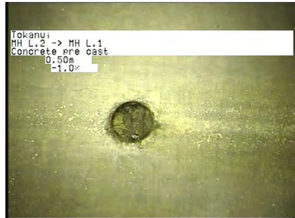
MH L.2 To MH L.1_20ebec42-80a7-4b70-bc9c-0acc7b94c2ef_20230328_113819_493.jpg, 00:00:28, 0.50m
