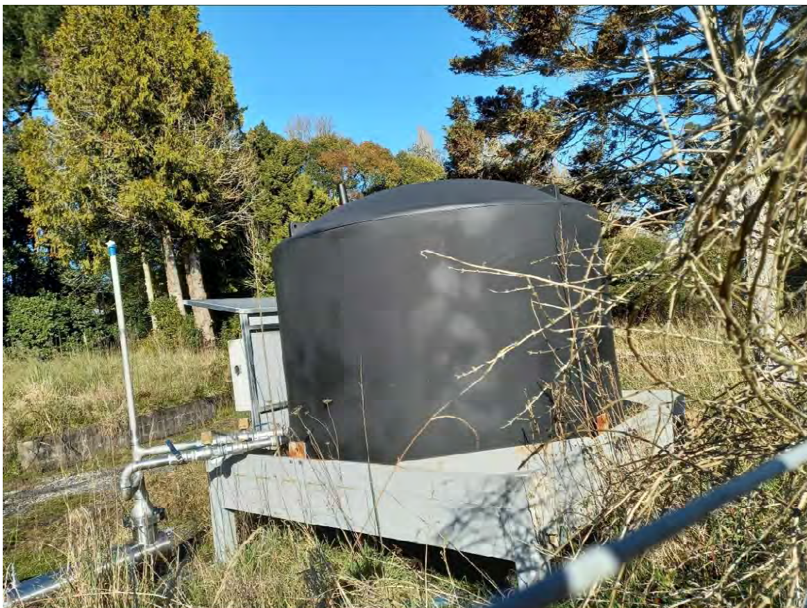
Figure 22: Redundant UV Treatment Plant
