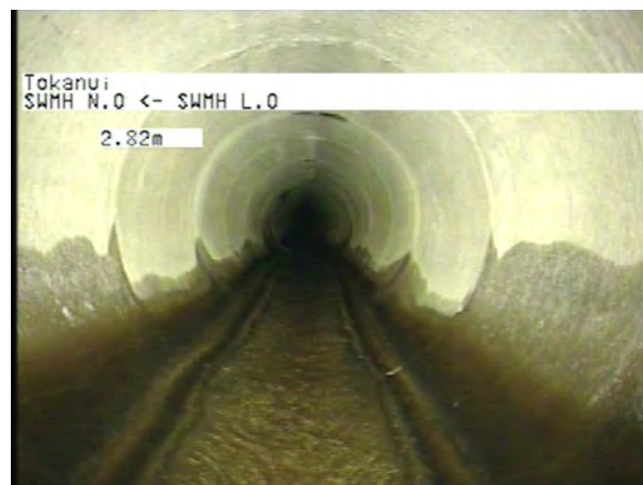
MH L.0 To MH N.O_bcd2da46-5308-4325-944e-bce3e7c063da_20230406_15 2657_067.jpg, 00:01:39, 2.82m
