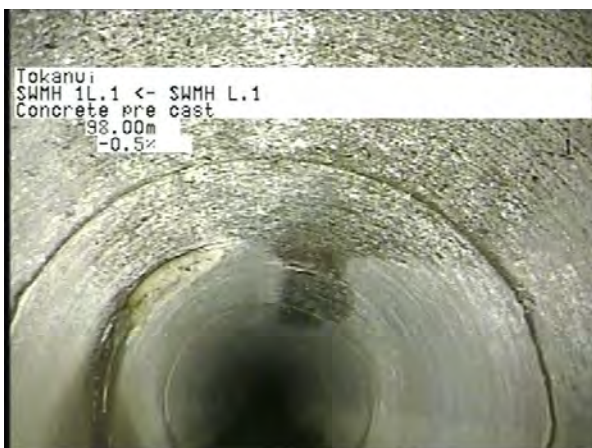
MH L.1 To MH 1L.1_c7b5bc8a-909f-4303-b4a7-2fb66a44ad2a_20230404_12 3203_411.jpg, 00:26:20, 98.00m
