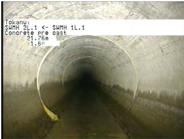
MH 1L.1 To MH 2L.1_f728b9c7-2735-4eb4-8496-00f25ba1a8e7_20230404_13 0019_167.jpg, 00:06:40, 21.76m
