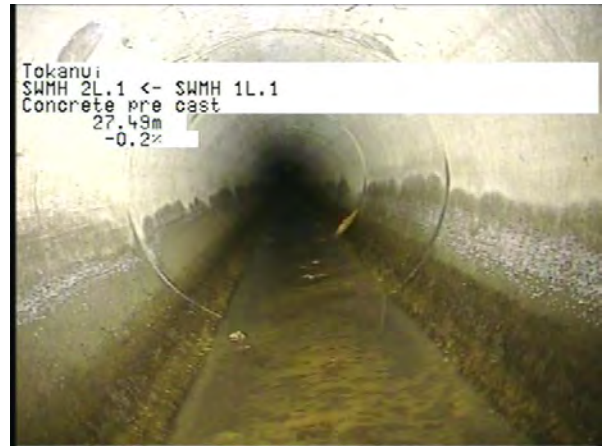
MH 1L.1 To MH 2L.1_87774ce4-2d50-4951-b680-e12bfc90df6a_20230404_13 0137_193.jpg, 00:07:51, 27.49m
