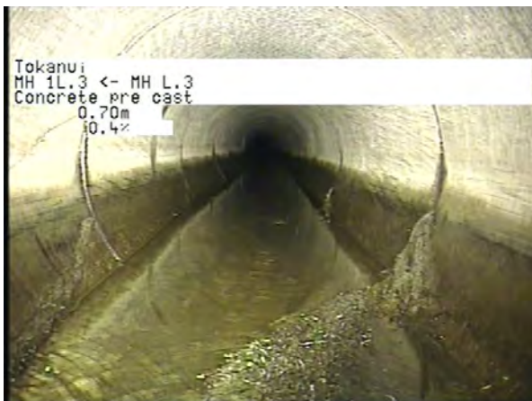
MH L.3 To MH 1L.3_3b63cc1a-fda2-4980-80ac-24fcff635840_20230404_102 957_802.jpg, 00:01:21, 0.70m
