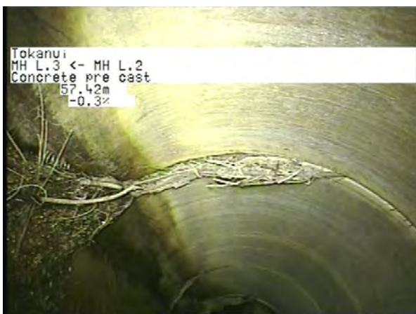
MH L.2 To MH L.3_03e73cab-167b-4032-b96d-6a3dc889c008_20230328_141144_508.jpg, 00:18:30, 57.42m
