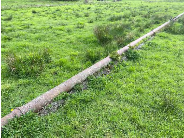
Pipeline situated on concrete foundation
