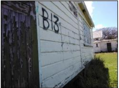
Page 175 of 255 Deteriorated building with lead-based paint
