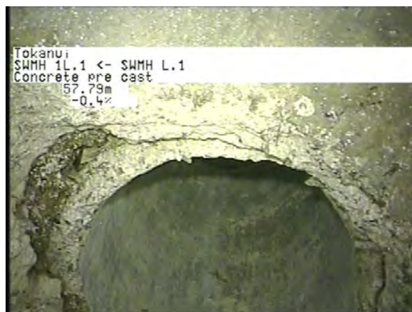
MH L.1 To MH 1L.1_42f8a8e7-9c5f-4050-acd7-894a60ad9256_20230404_12 1758_258.jpg, 00:15:44, 57.79m
