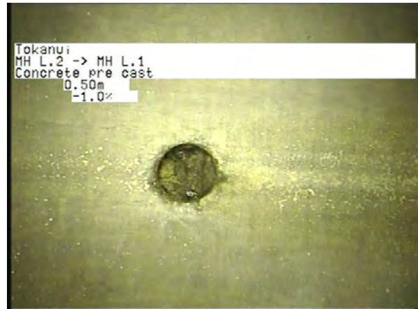
MH L.2 To MH L.1_20ebec42-80a7-4b70-bc9c-0acc7b94c2ef_20230328_113 819_493.jpg, 00:00:28, 0.50m
