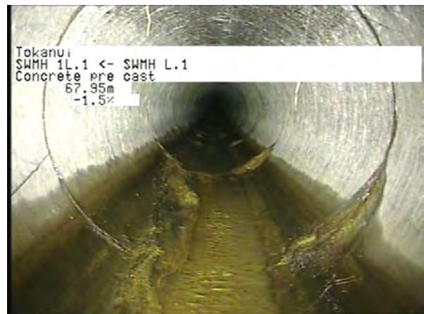
MH L.1 To MH 1L.1_510fc2ed-e598-4f17-88f0-a68e8f3b1666_20230404_122 316_895.jpg, 00:19:02, 67.95m
