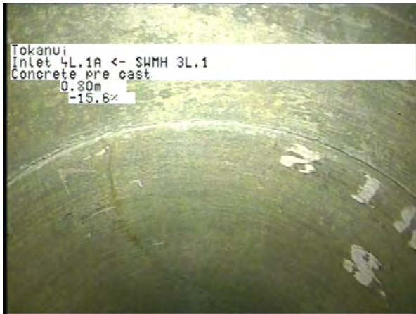
MH 3L.1 To 4L.1A Inlet_6e2fd88e-489a-4334-925a-5ea1c237ff7c_20230406_14 2434_799.jpg, 00:00:36, 0.80m
