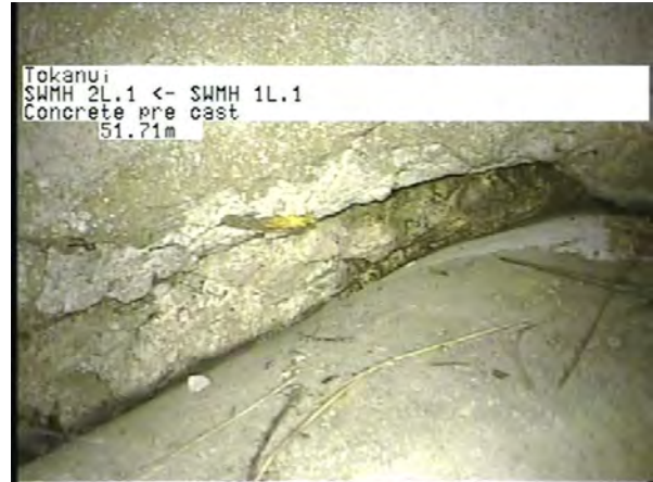
MH 1L.1 To MH 2L.1_b4f8d65b-9a35-42c1-bc8c-fb426e3f6133_20230404_13 0841_954.jpg, 00:13:37, 51.71m
