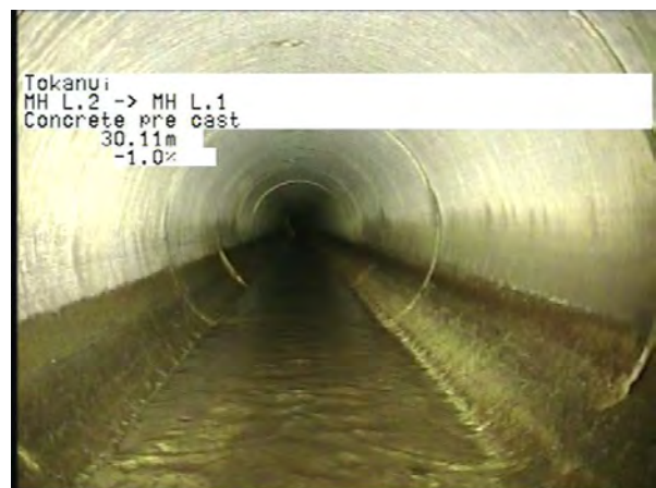
MH L.2 To MH L.1_ecea2b43-d4e0-4411-be2f-42ea484c9973_20230328_11 4733_026.jpg, 00:08:38, 30.11m
