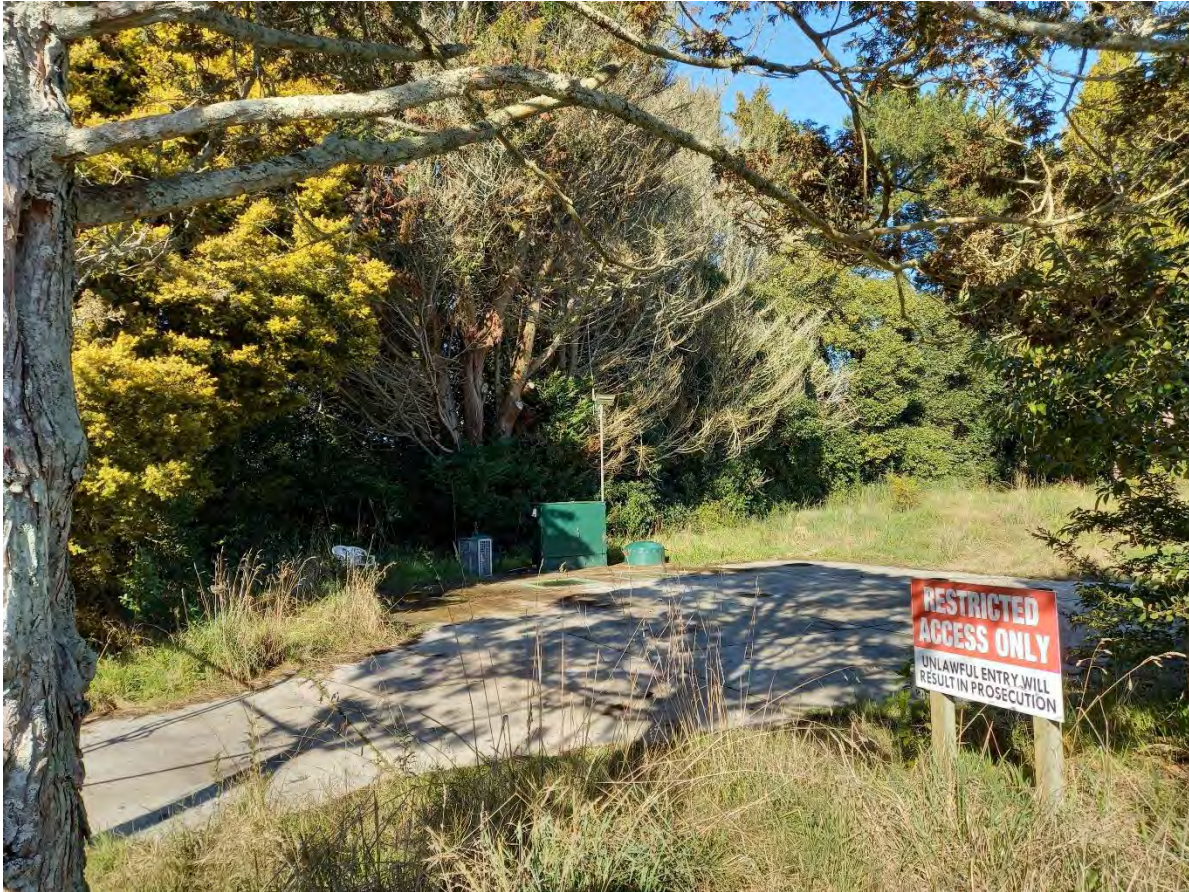
Figure 19: New Wastewater Pump Station (in ground tanks and chambers under concrete pad)
