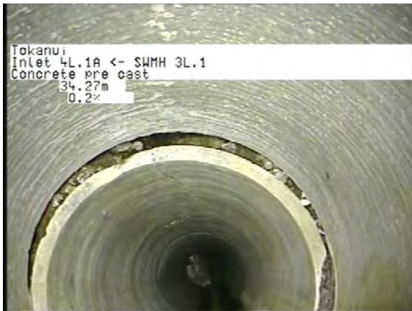
MH 3L.1 To 4L.1A Inlet_0f017929-4dd3-4872-8303-7d38d6cd798e_20230406_1 43407_948.jpg, 00:08:17, 34.27m
