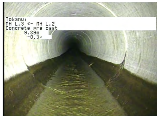
MH L.2 To MH L.3_838cbd75-93b0-4437-922b-ec6b662c3dd9_20230328_13 5257_735.jpg, 00:03:45, 9.89m
