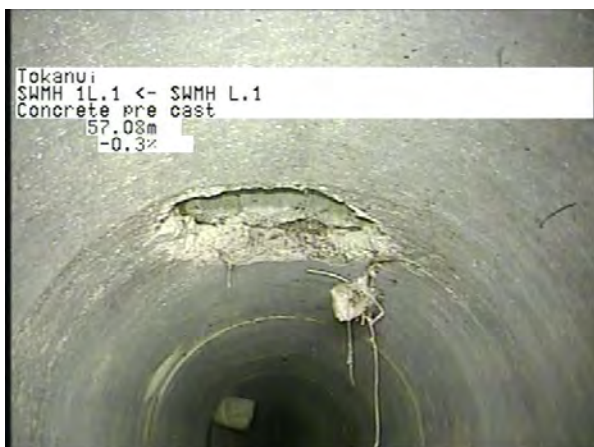
MH L.1 To MH 1L.1_86a0788c-11dd-40f7-a6c0-3777bbc11132_20230404_1 21725_361.jpg, 00:15:28, 57.08m
