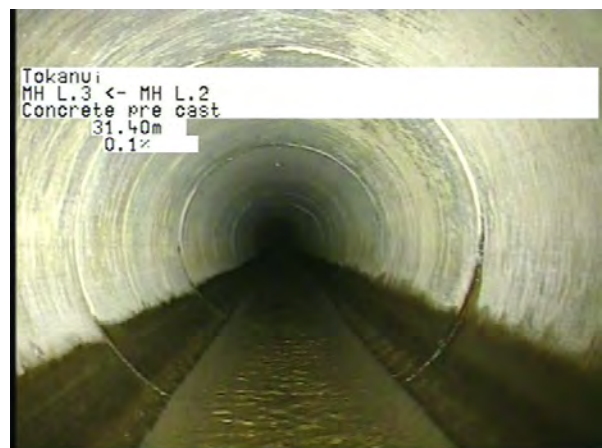
MH L.2 To MH L.3_0167836e-dc1a-4ab9-8c15-90217fcd2ad6_20230328_14 0015_663.jpg, 00:09:40, 31.40m
