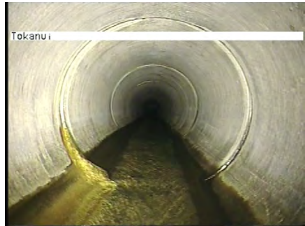
MH L.3 To MH 1L.3_735a4276-00cb-4f96-888d-98baefb8c386_20230404_10 5617_608.jpg, 00:23:54, 89.18m
