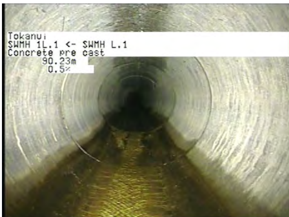
MH L.1 To MH 1L.1_0f5006bf-4117-4fb8-bc62-3c18a0844030_20230404_12 3000_556.jpg, 00:24:42, 90.23m
