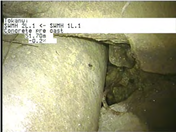
MH 1L.1 To MH 2L.1_d2d5e66b-6c21-4dc5-809b-275de36f7b36_20230404_1 30832_089.jpg, 00:13:37, 51.71m
