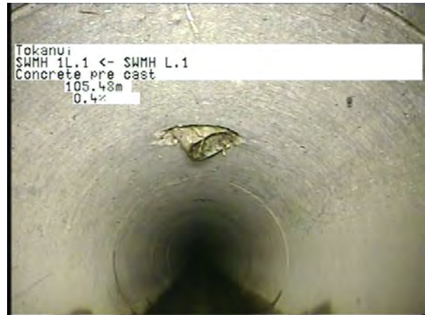
MH L.1 To MH 1L.1_2c7ef29f-c7e1-41ca-ae0c-a44b80309301_20230404_12 3504_608.jpg, 00:28:56, 105.48m
