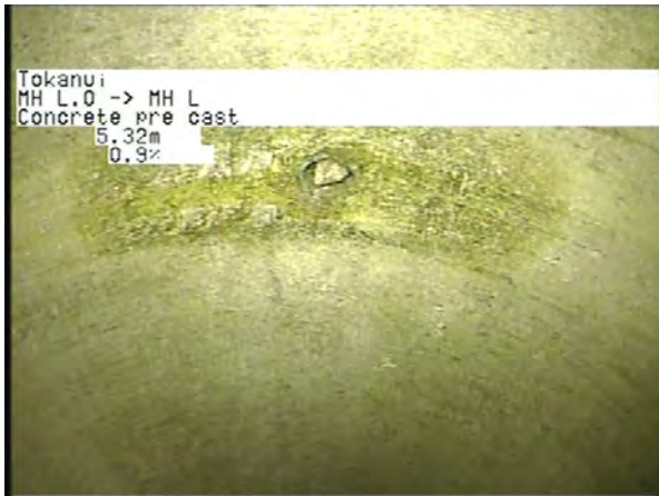
MH L.0 To MH L_bc5c82b4-6374-44e7-a6f7-cb496a6223fa_20230328_122801_777.jpg, 00:01:23, 5.32m
