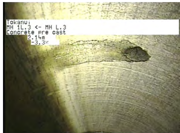
MH L.3 To MH 1L.3_8f3149b8-46b5-47b3-a989-f6b5b56313f4_20230404_10 3057_801.jpg, 00:02:15, 2.14m
