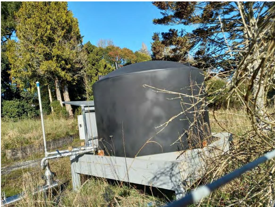
Figure 22: Redundant UV Treatment Plant
