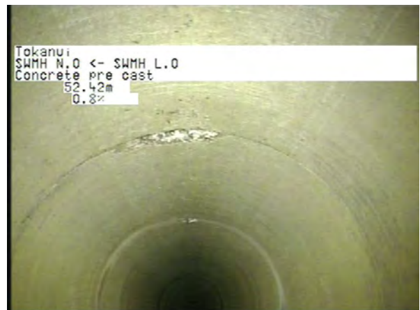
MH L.0 To MH N.0_f1a43aad-f720-4bba-89eb-06cf6aa0544d_20230406_153 541_152.jpg, 00:09:21, 52.42m
