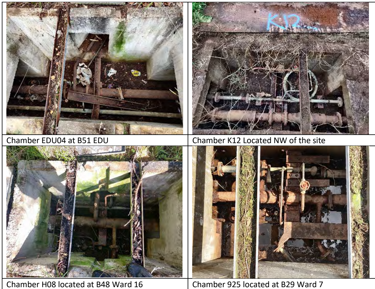
Figure 13: Representative Photos of the Concrete Ducting System
