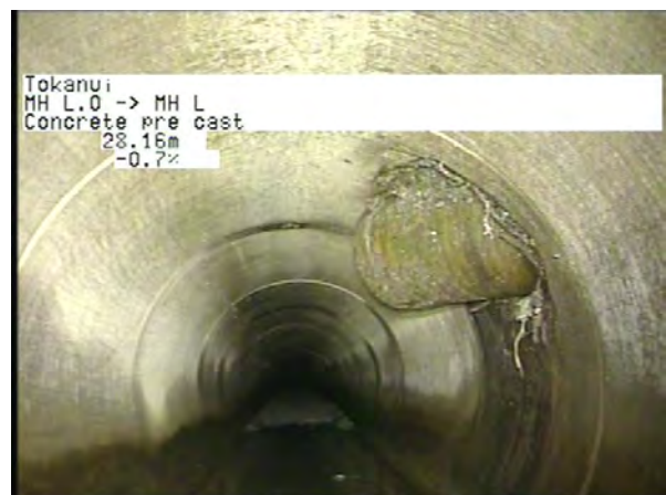
MH L.0 To MH L_ddd0d91a-fb41-455c-ab15-3b164221f884_20230328_123445_310.jpg, 00:07:15, 28.16m
