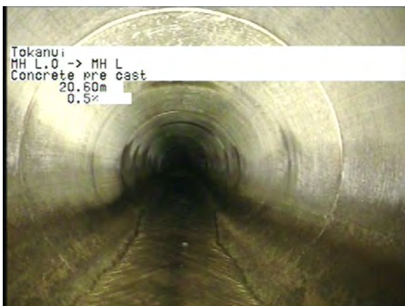
MH L.0 To MH L_0e8bd76d-7a14-4391-8c30-2cdb63caf836_20230328_123306_887.jpg, 00:05:45, 20.60m
